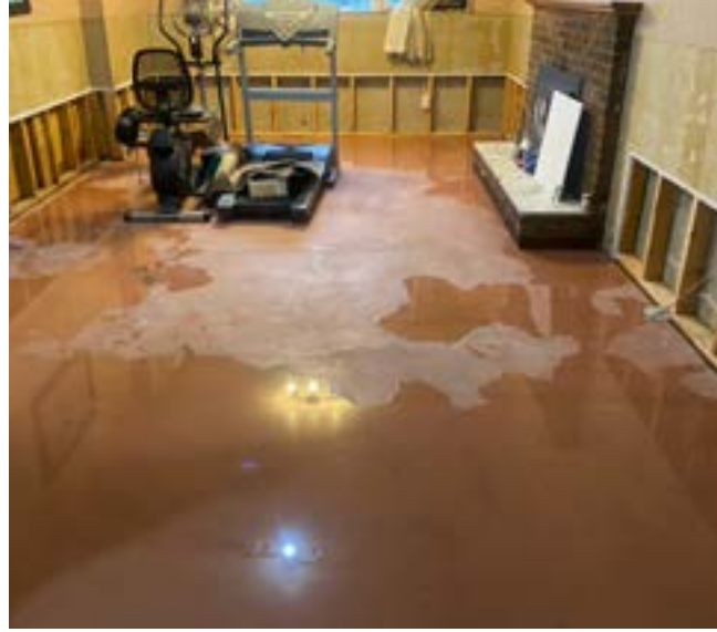
Flood damage in our second stage housing in November, 2021
